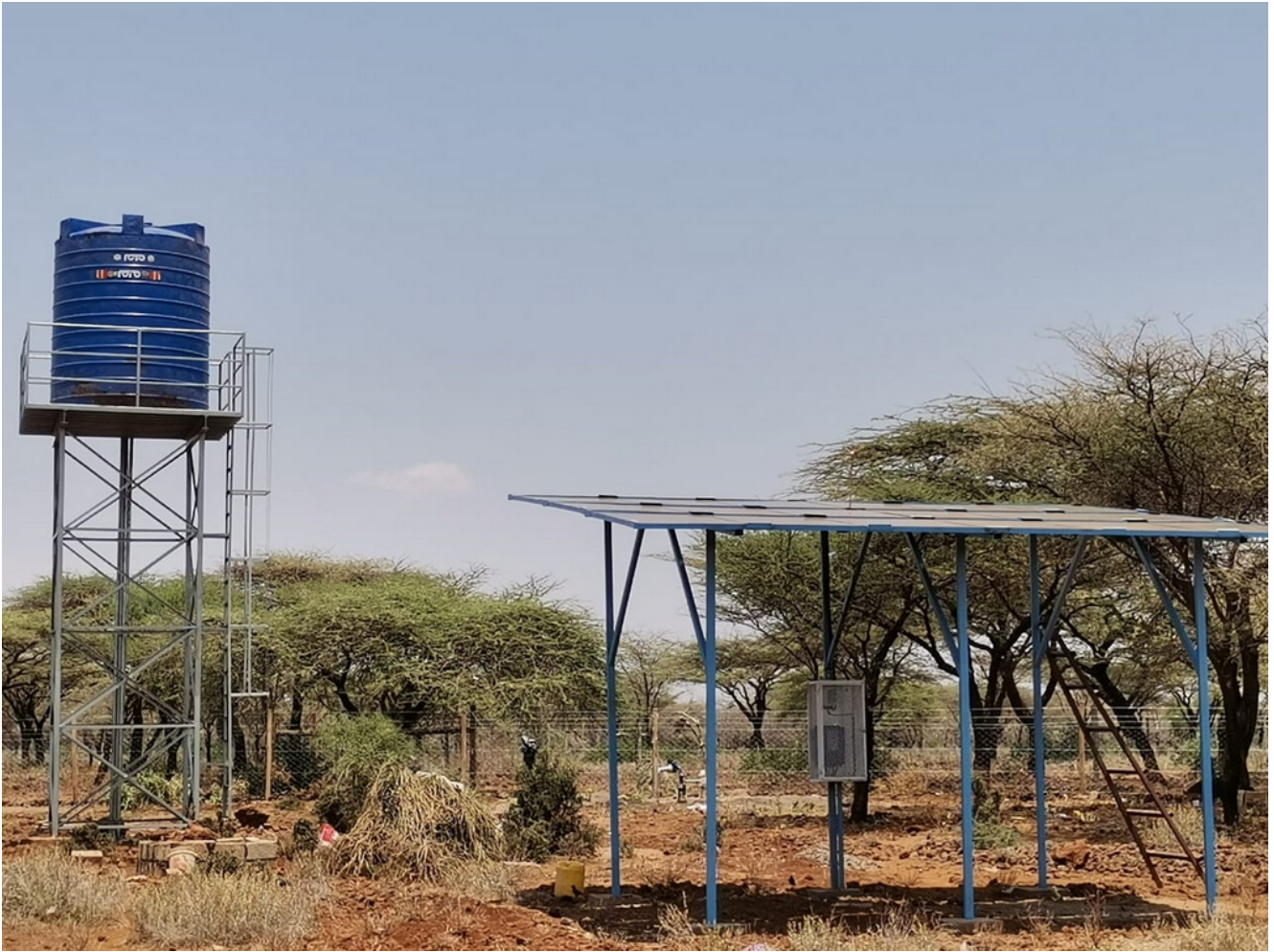
Chumviere Boreole – Isiolo – water tank and solar panel
